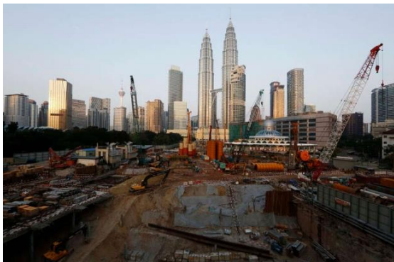
A file picture of a construction site next to the Petronas Towers in Kuala Lumpur. A prominent economist says the nation has been paying less attention to real economic indicators such as the future of agriculture as well as de-industrialisation. — Reuters pic
